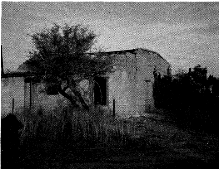
Figure 2. This photo shows one of the original officer's quarters at Fort Lowell. The building was built in 1873. The original adobe bricks and the stucco finish are both apparent.
