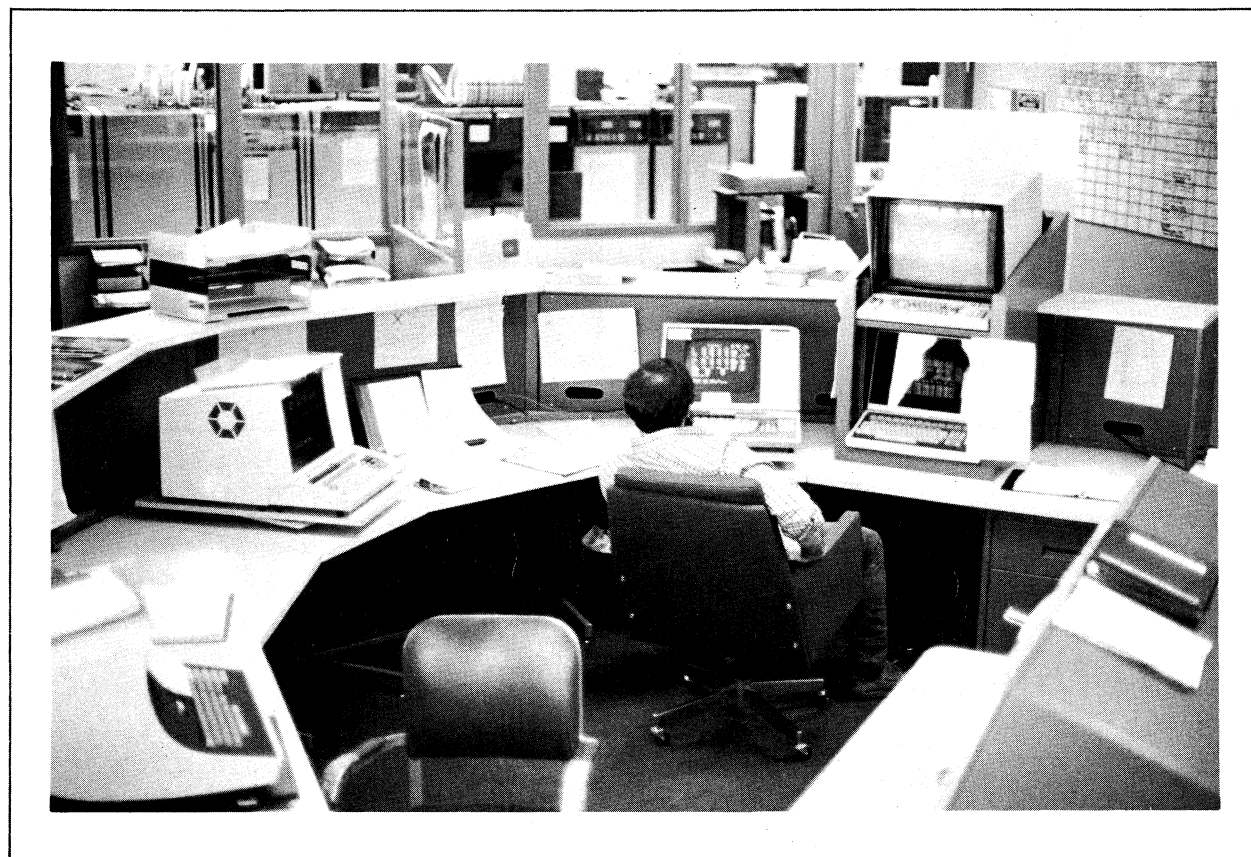
Figure 4-1. A photograph of the array control room, with an array operator sitting amongst on-line and off-line communication terminals. The computer room is seen through the windows to the rear. Some of the on-line computer system MODCOMPS are visible just beyond the windows, and portions of the off-line computer system are seen in the background.
