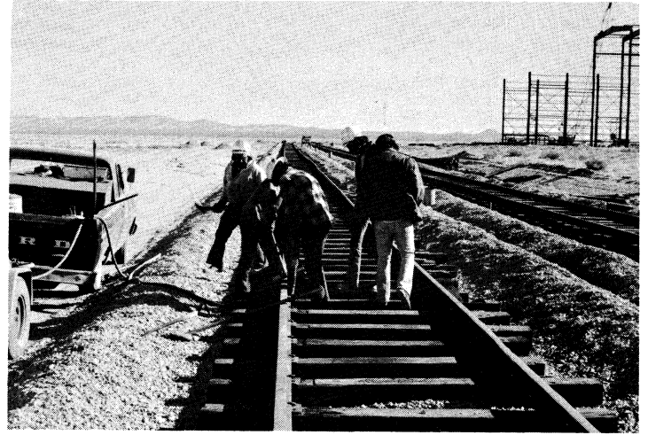
Spiking and preliminary alignment of the track. Upper right: portion of the Antenna Assembly Building.
