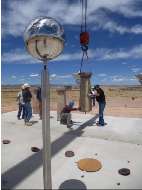
Fig. 32. A pier is gently lowered into place by a crane. Photo: Sullivan.
