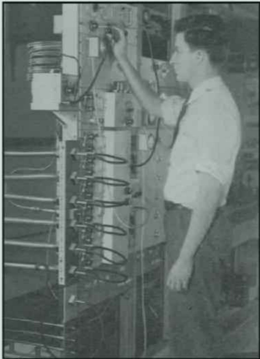
Fig. 17—View showing the six transmission lines and coaxial patch cords . The beating oscillator is mounted upon the shell and is connected to the power amplifier (which is being adjusted by Mr. Edwards) at the top of the bay.
