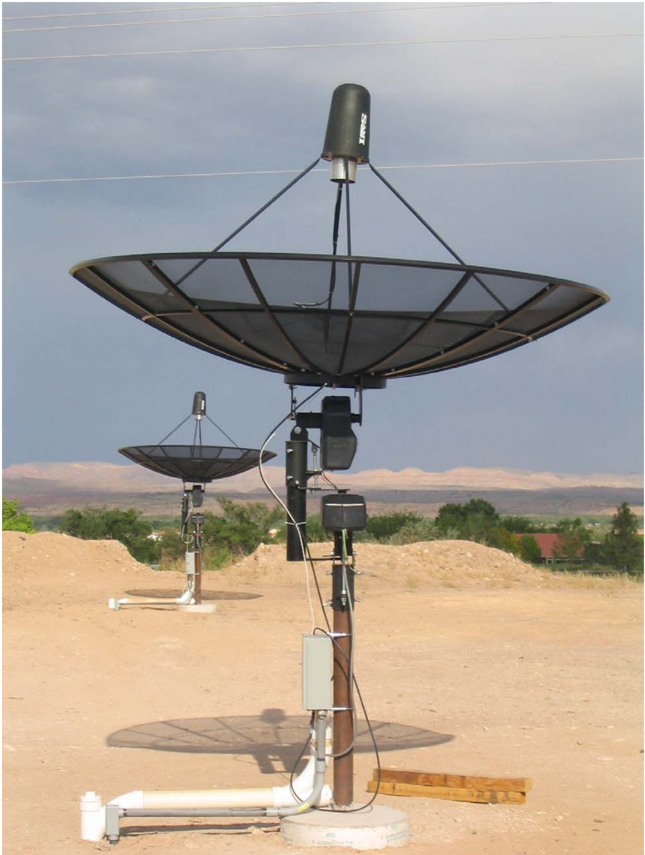
Fig. 5.— The two ten foot radio dishes spaced 24 meters apart.
