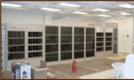
Figure 3. The first quadrant of the bilateral correlator that will eventually link 64 antennas has been installed in the AOS Technical Building.
