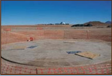
Figure 1. A concrete AOS antenna foundation cures. Cerro Chico is in the right foreground. Photo by Patricio Pardo.
