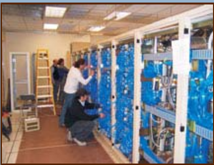
Figure 3. One thousand three hundred cables have been installed in the first correlator quadrant in its oxygenated AOS technical building home. Automated software detected two interchanged cables, which were quickly corrected.
