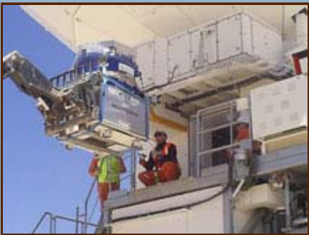
Figure 2. The first ALMA production Front End is guided into the receiver cabin on Melco antenna No 2.
