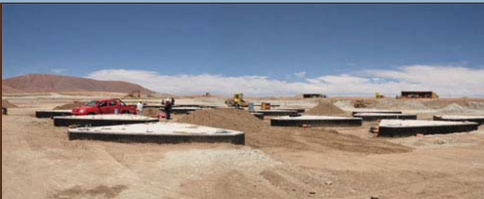
Figure 2: Construction continues on the foundations for the Atacama Compact Array. The foundations for the 7m antennas, shown here, allow the antennas to be spaced 8.75m apart.
