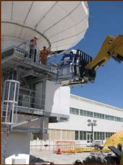
Figure 1: By mid-February, the newly accepted Vertex antenna had been outfitted with ALMA systems. In this photo, a Front End system is being loaded into the antenna receiver cabin.
