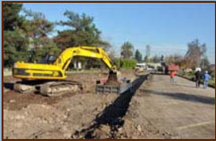
Figure 2: Excavation has begun on the new Santiago Central Office for the Joint ALMA Observatory, adjacent to the ESO offices in Vitacura. © ALMA (ESO/NAOJ/NRAO)
