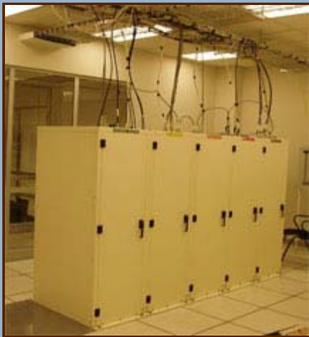
Figure 2. The ALMA Central Local Oscillator has been successfully installed at the 5000m AOS Technical Building. Photo: W. Grammer.
