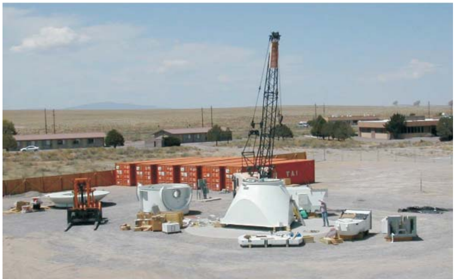
Assembly of the VertexRSI antenna has begun at the ALMA Test Facility (ATF) located on the VLA site.
