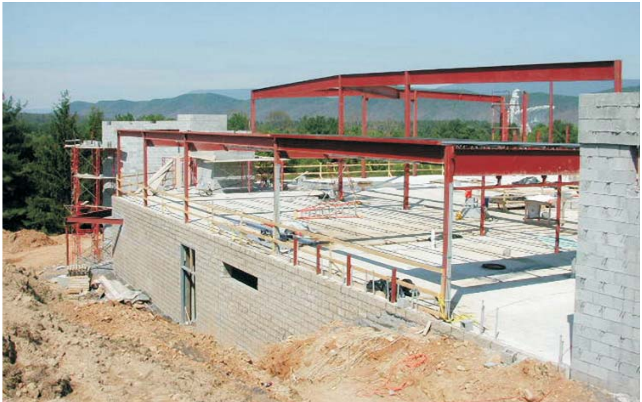
The Green Bank Education and Visitor Center construction continues to be on schedule. Here the exterior construction of the lower floor, the lower floor masonry work, the upper floor slab, and the steel superstructure for much of the upper floor are visible.
